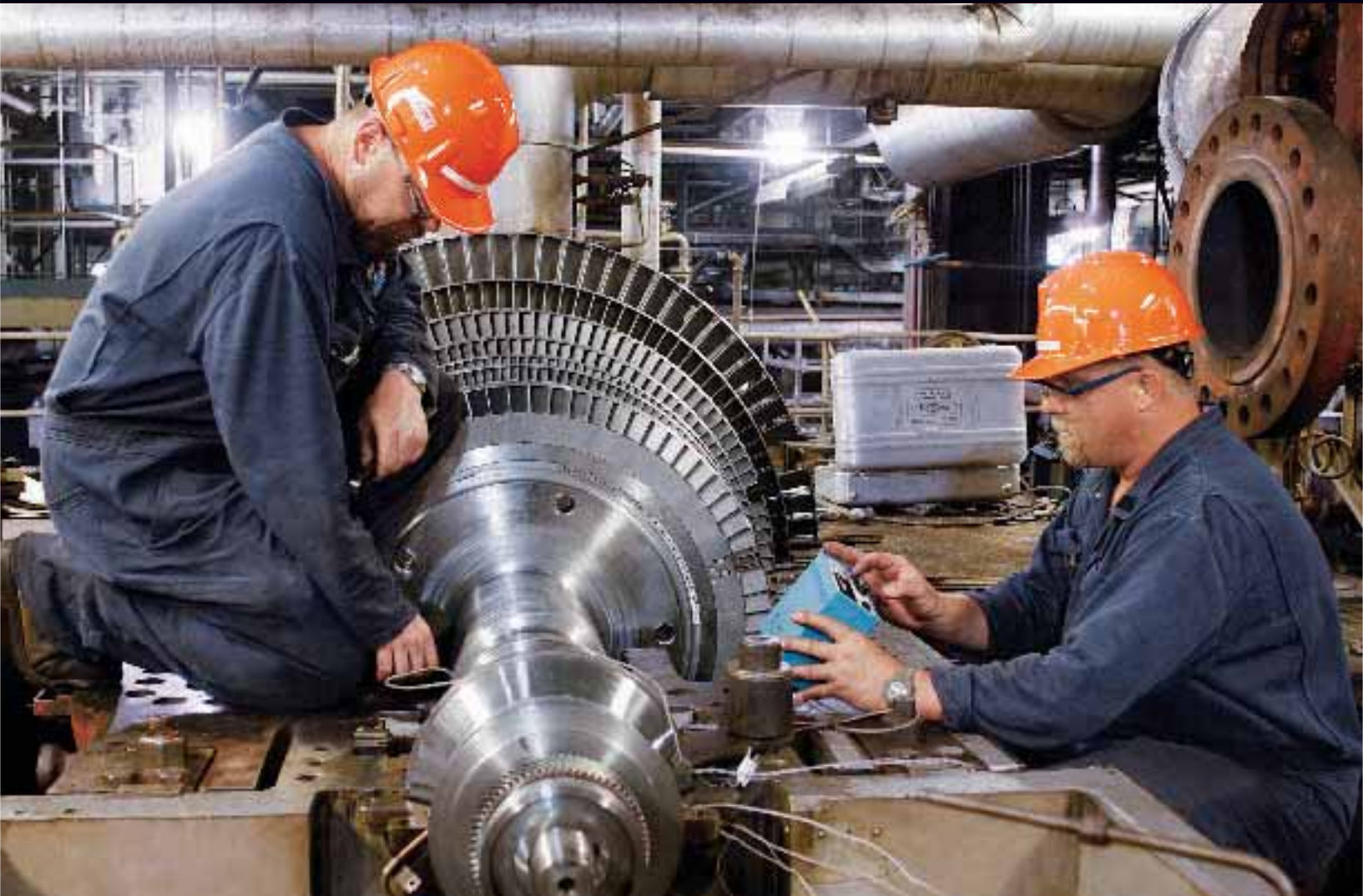
OPG employees retrofit a new boiler feed pump at the Lambton fossil-fuelled station
