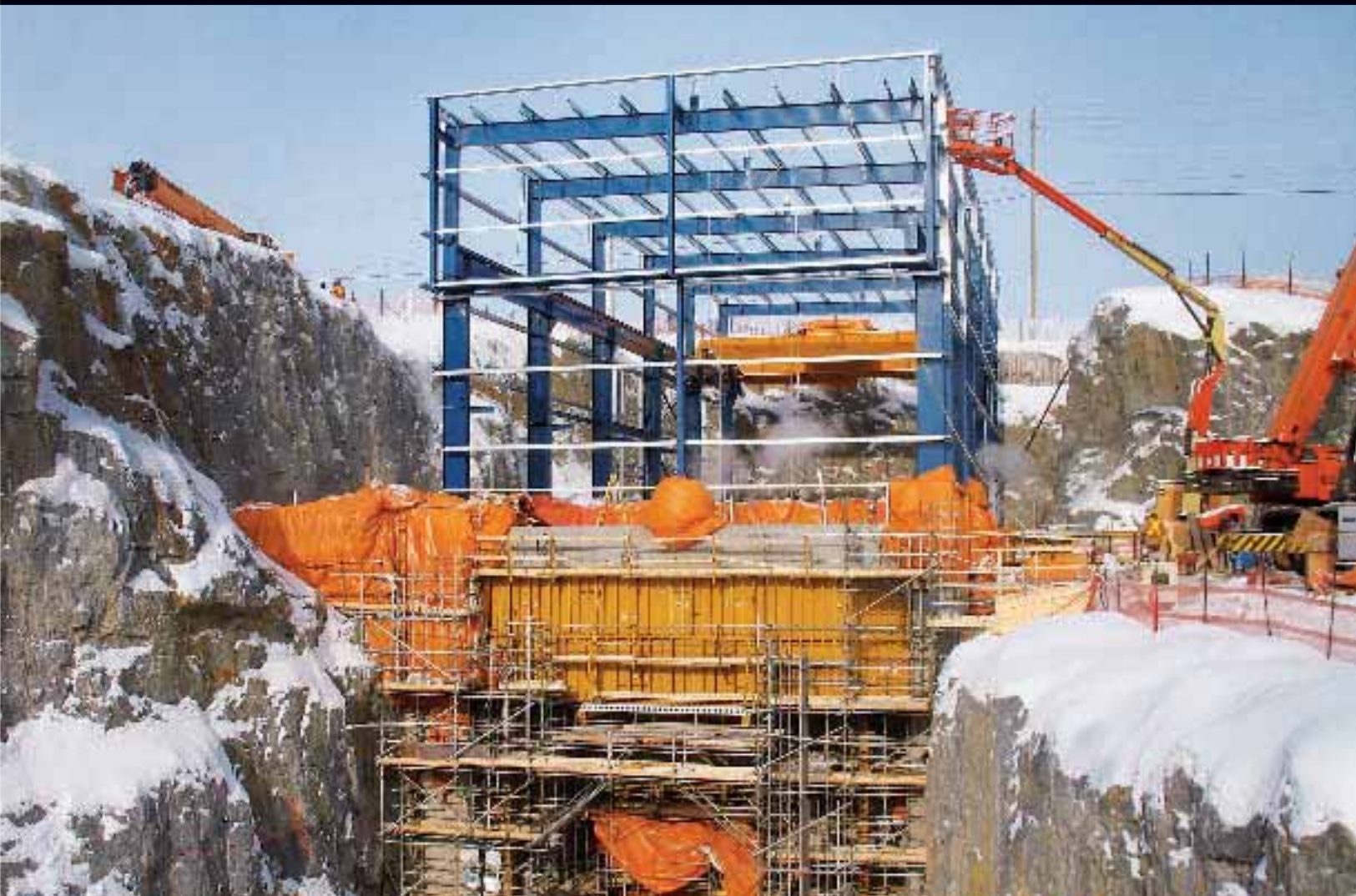
OPG's 12.5 MW Lac Seul hydroelectric generating station, under construction in Northwest Ontario
